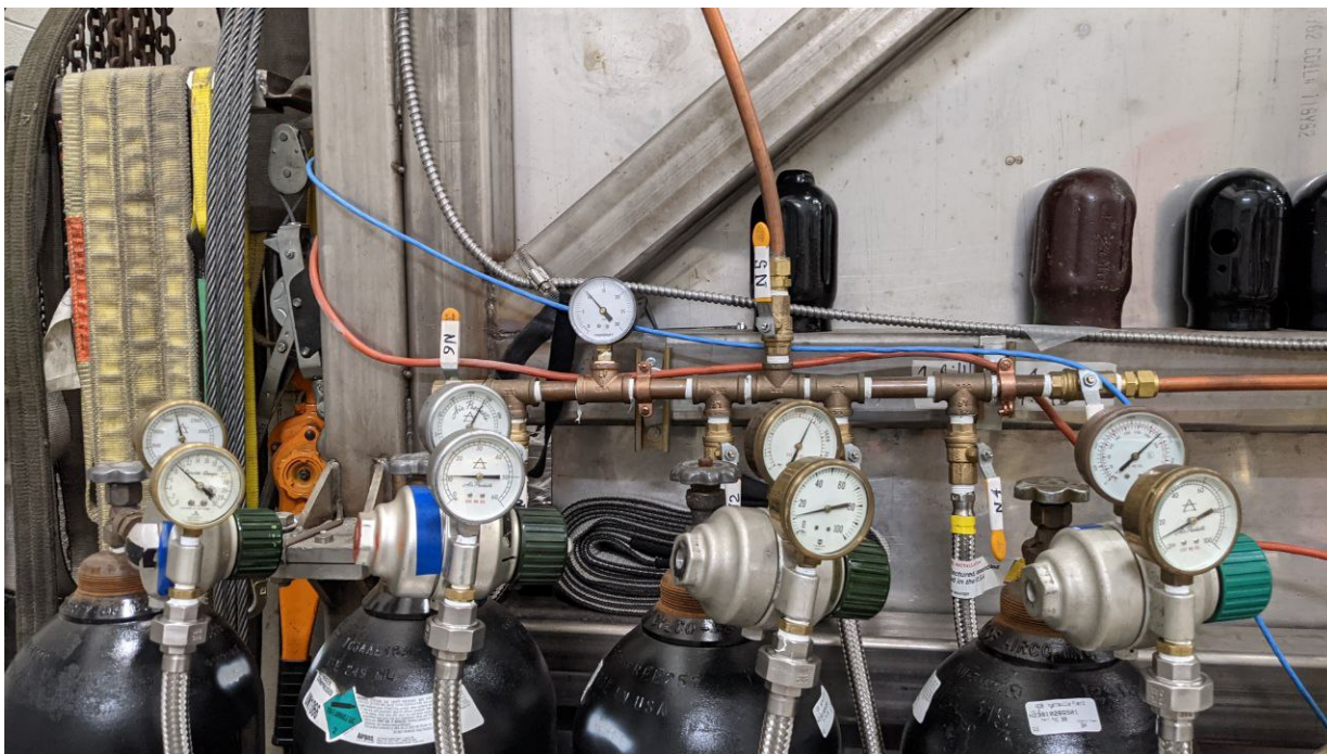
Figure 3.12: The picture of the nitrogen high flow pressure system main hub.
