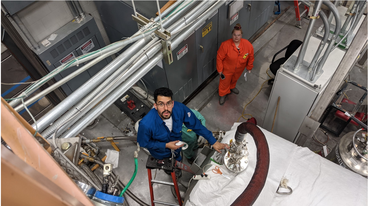
Figure 3.25: Rubén Rojas adding the heating tape to the valve to heat up and liquefy solid sodium inside the transfer line valve during the refilling operation.
